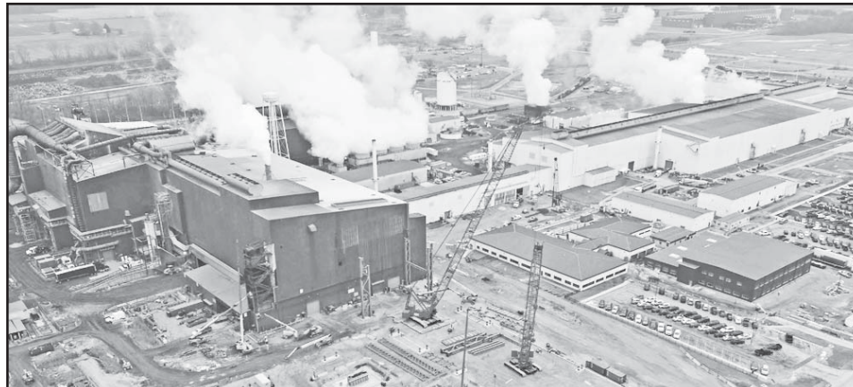
The project has a special focus on supporting the increased electricity needs of North Star BlueScope Steel for the $700 million expansion project of its steel mill in Delta
