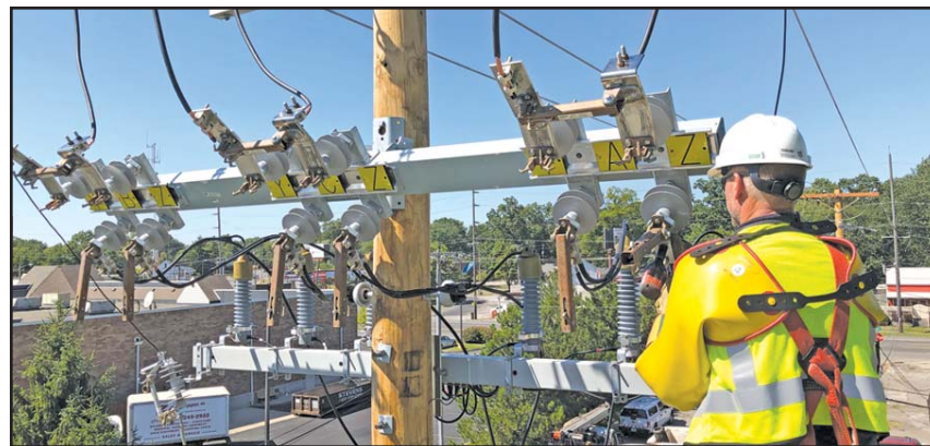
Toledo Edison's project has additional investment being placed in technology modernization and tree trimming
