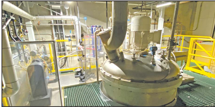
Lubrizol's expansion enables the company to produce more surfactants
