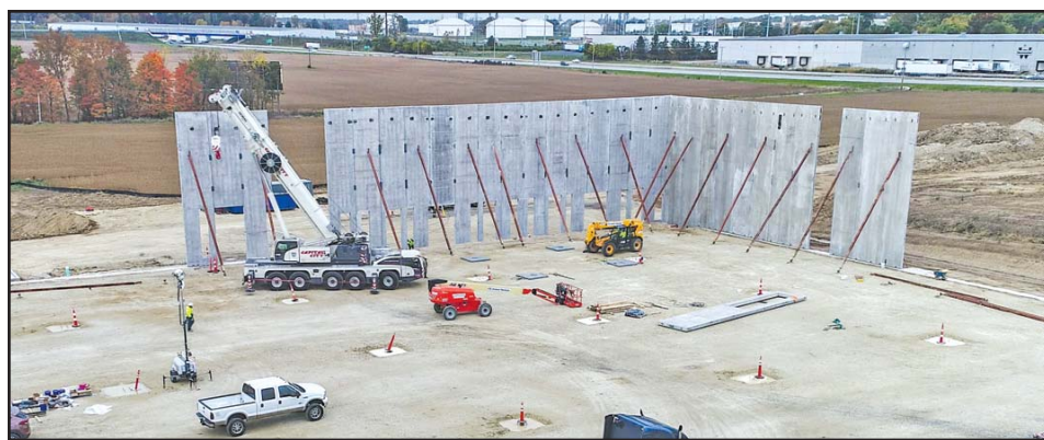
Walls are going up on the new Logoplaste facility in Lima's Gateway Industrial Park
